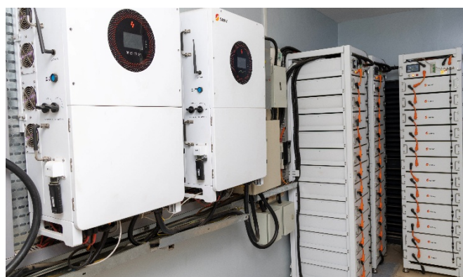
Kandia’s inverter and solar batteries
