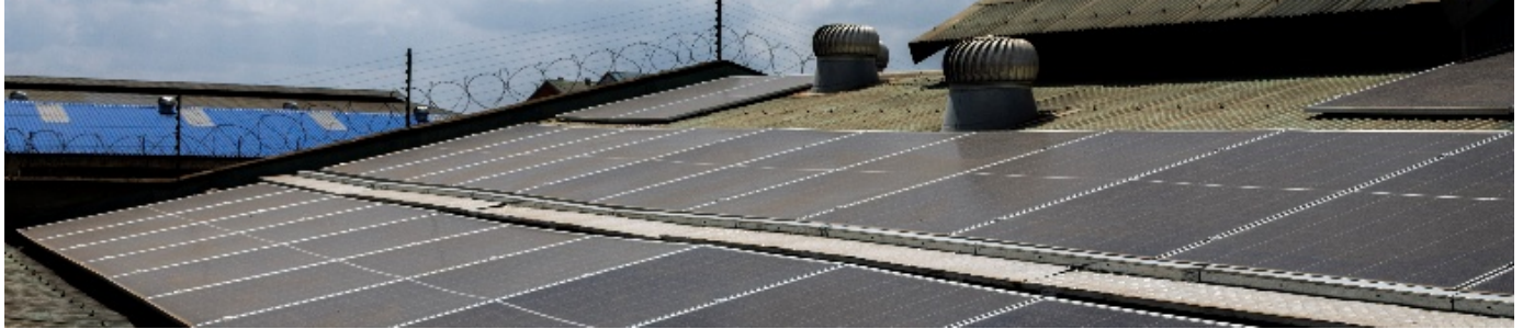
Solar panels installed at Kandia Fresh Produce Suppliers Ltd.
